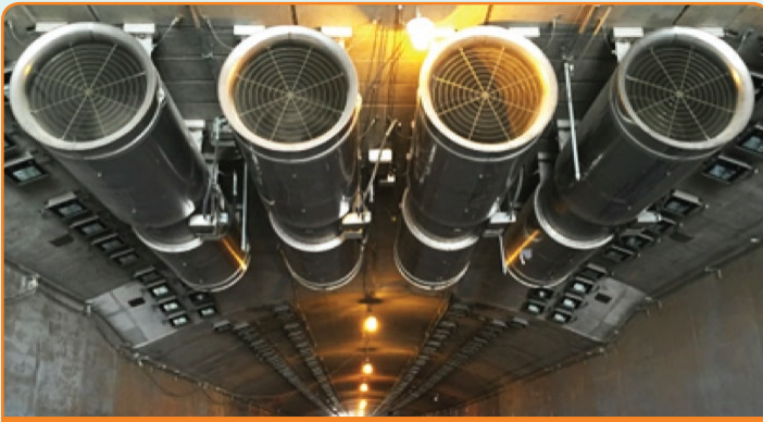
Tunnel Jet Fans
